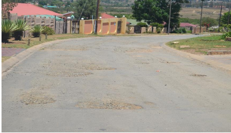
one of the streets needs to be resurfaced by KSD (Nombembe str)
